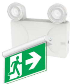
Emergency Exit Lighting
